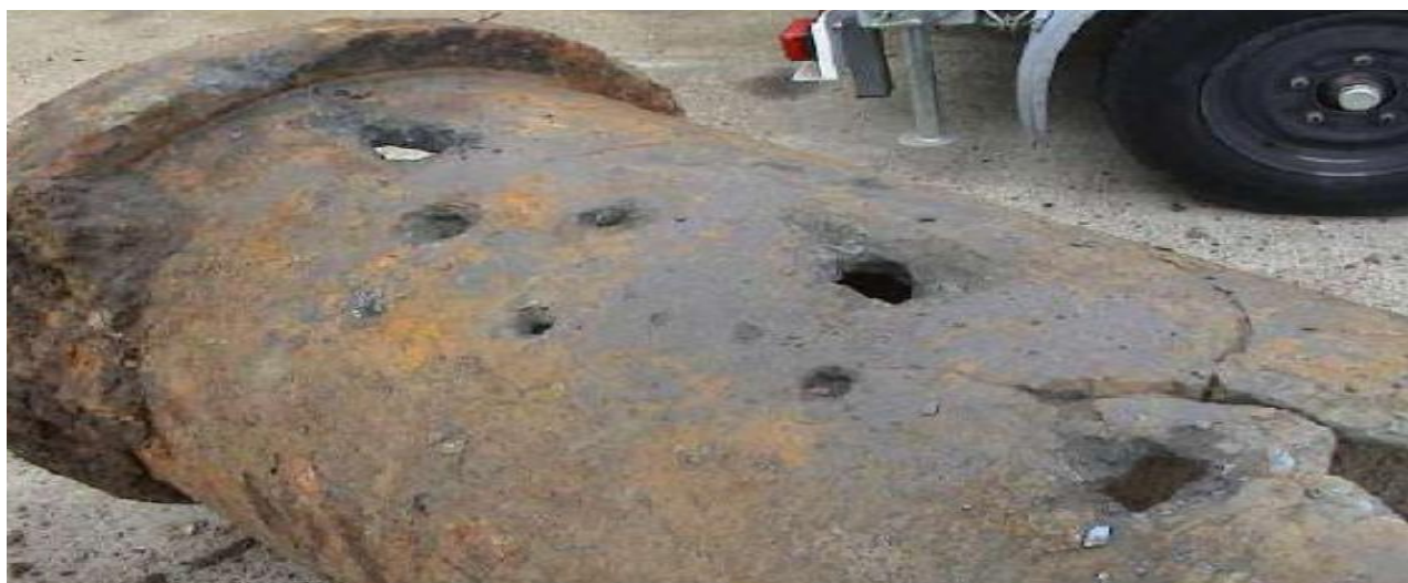
Figure 5 – Evidence of asset condition deterioration of Conduit 3 main. Teesside Strategic Network Study, 2017
