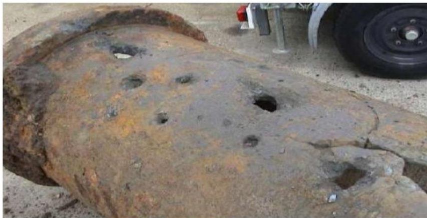
Figure 34 – Evidence of asset deterioration of T4 main, Darlington
