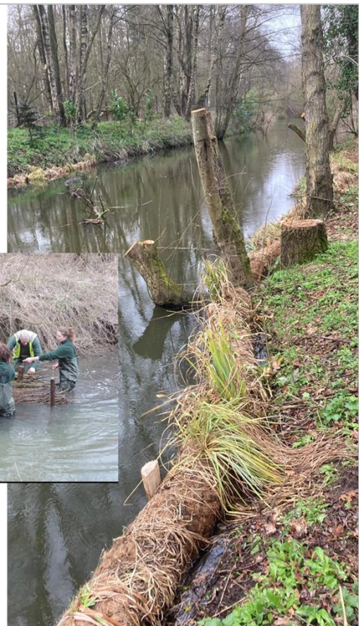
Businesses visited in Diss as part of the Yellow Fish Campaign and installation of flow deflectors and coir matting
