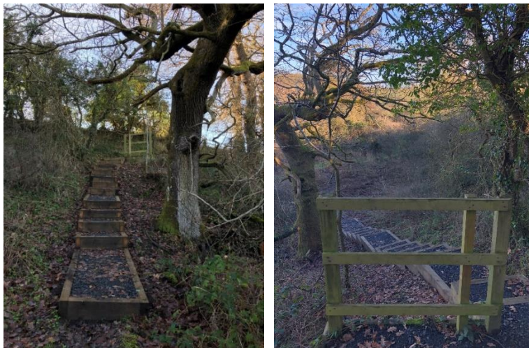
New steps and handrail at Ulgham Local Nature Reserve delivered in kind by local contractor following NRT assessment
