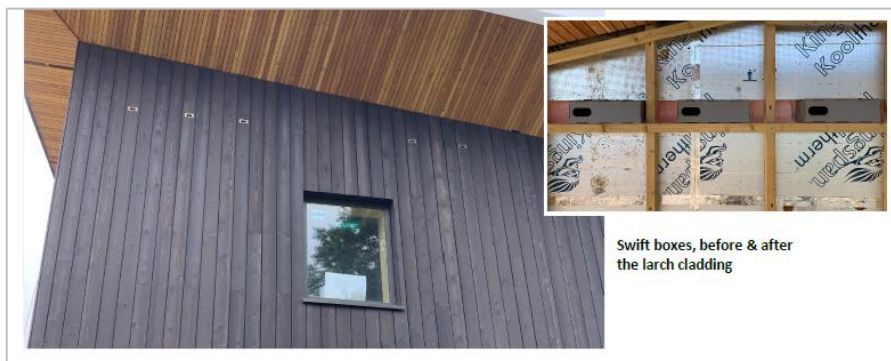
Swift boxes created into the cladding of the visitor centre (taken from SWT annual report for Branch Out)
