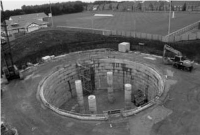
Waste water storm tank, South Shields, part of our £3.0 million flood alleviation scheme
