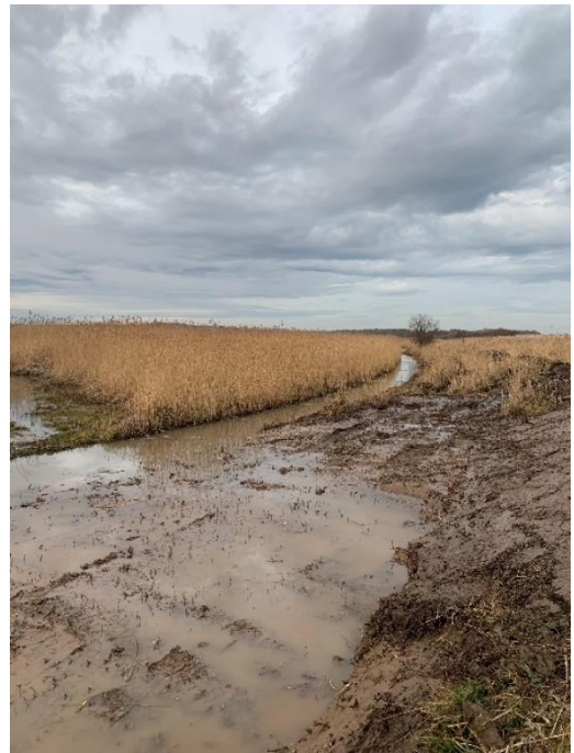
Re-exavated drainage ditch and wet mud scrape to enhance and create micro habitats but also provide different viewing areas for wildlife watchers (a month after this work was completed a Water Rail was spotted)
